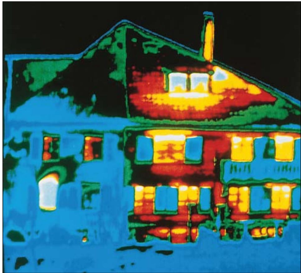
Thermal image showing energy leakage from building.
